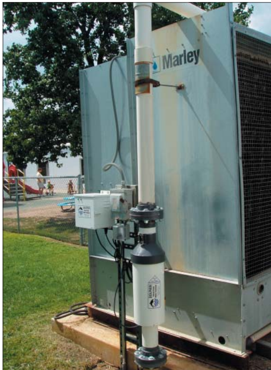
Photo: Clearwater Systems Corporation
