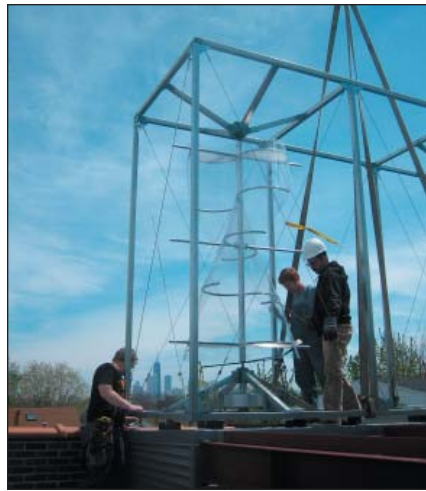
Workers install one of three wind turbines on the roof of a renovated mixed-use building in Chicago. Photo: Brian Peters
