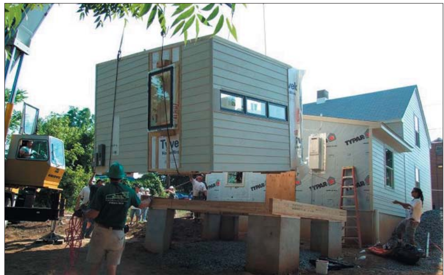
A small module, designed and built by EcoMOD students, is lowered onto its foundation in Charlottesville, Virginia. A module added to the historic house in the rear, along with the module in motion, added affordable housing units to the market.
