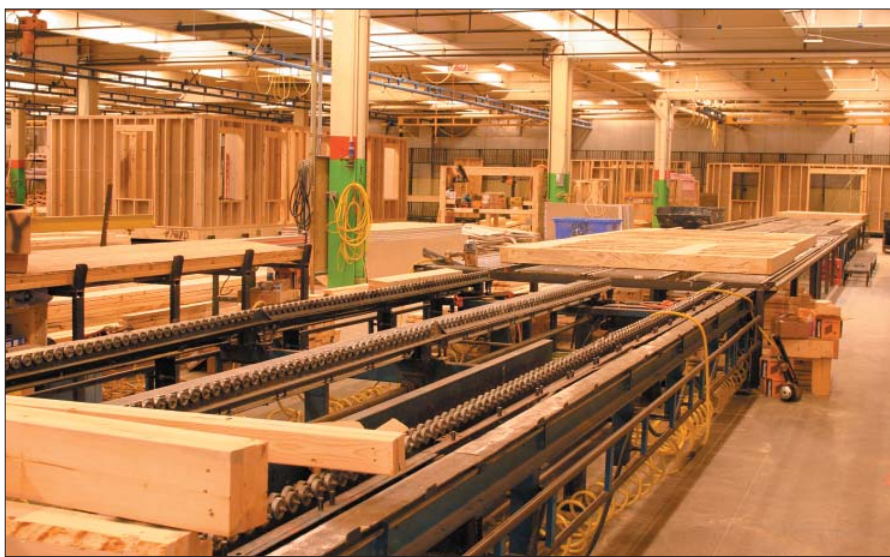
At the beginning of the assembly line at Customized Structures in Claremont, New Hampshire, walls are built and squared on special tables. They are then put on floor assemblies to create modules, shown at the rear on the left.
