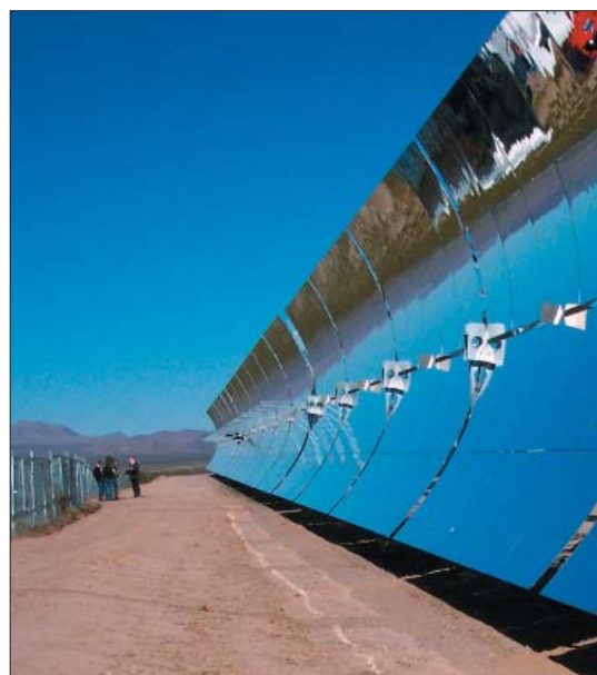
The Nevada One solar power plant, located in Boulder City, Nevada, is the third-largest plant in the world, providing 64 MW of electricity. Photo: Acciona Solar Power
